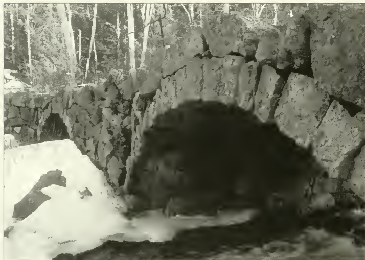
Above: The double-arched Carr Bridge in Hillsborough, New Hampshire, is a remarkable example of dry masonry stone work. A double-arched bridge allows for the necessary volume of water to flow through and still keeps the height of the bridge consistent with the roadbed. The granite was probably cut from deposits right by the river. Photo by Lynn Martin
